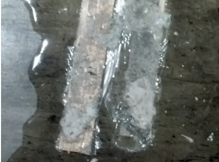
(A) Picture of broken concrete
