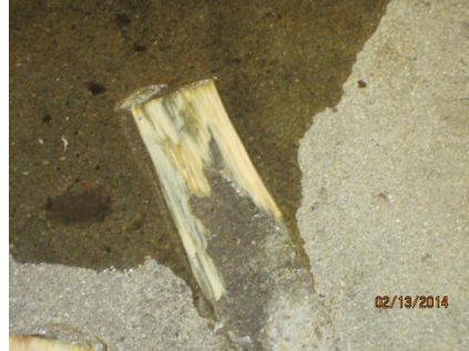
(B) Picture of broken wood
